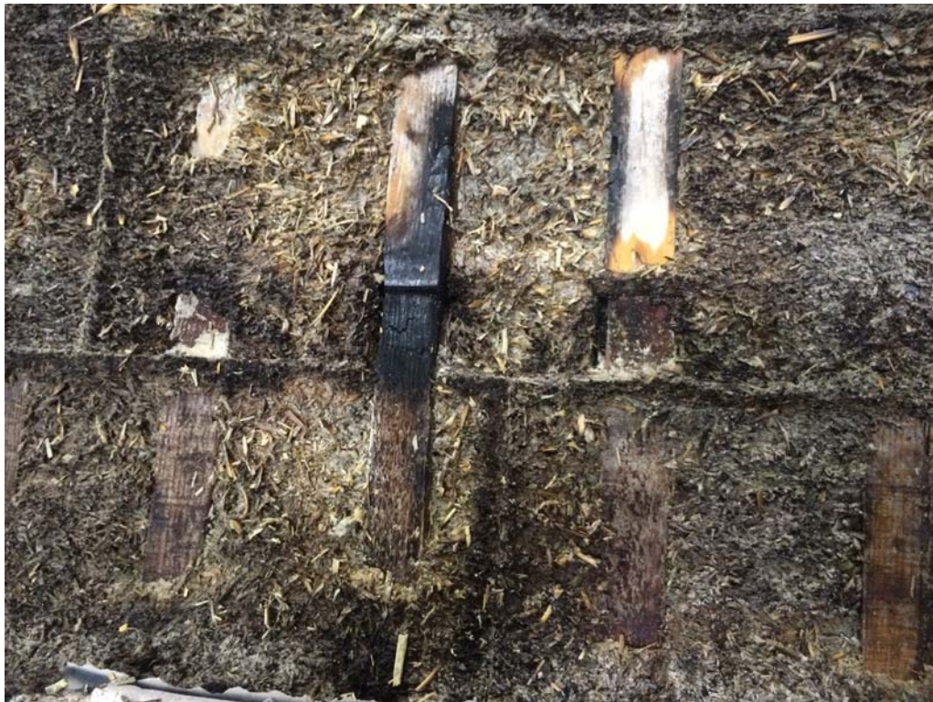
Figure 12: Exposed side after hose stream test at the center lower portion of wall near the area where the plaster had fallen off.
